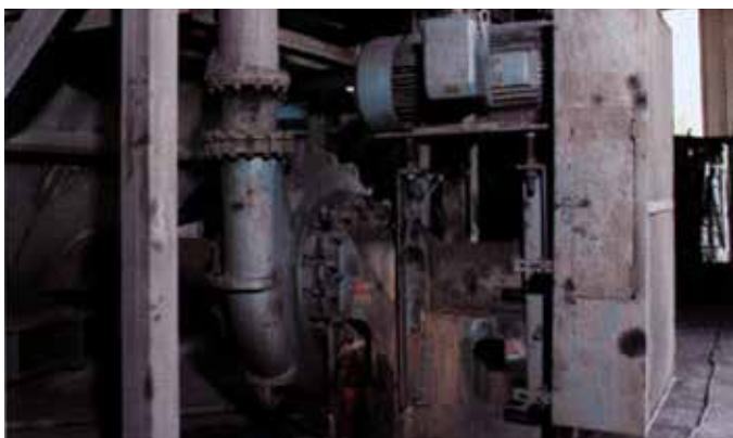
Overhead motor-mounted Model 5500 in a coal preparation plant – heavy media cyclone feed service.
