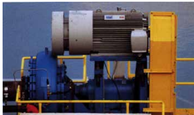
Model 5500 with 450 HP motor-mounted overhead on gold tailings reclamation service.
