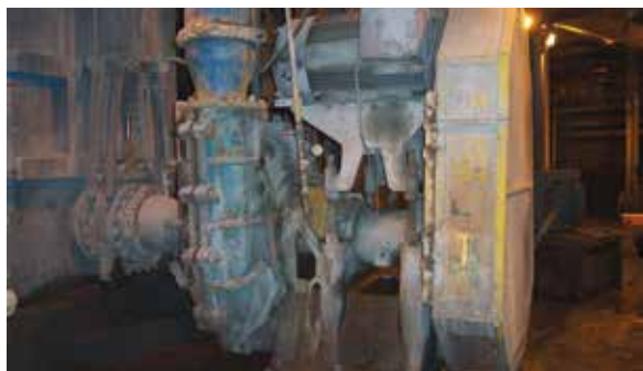
SRL-XT 14×12–36 on Ball Mill Discharge Service
