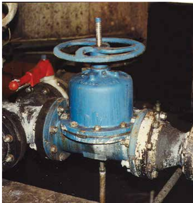
Straightway Valve on Abrasive Slurry Service
