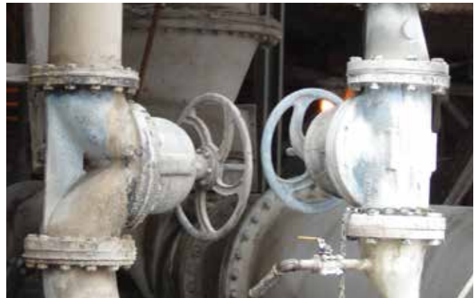
Weir Type Valve in Phosphoric Acid Service
